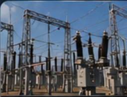
UTILITY & POWER GRID
